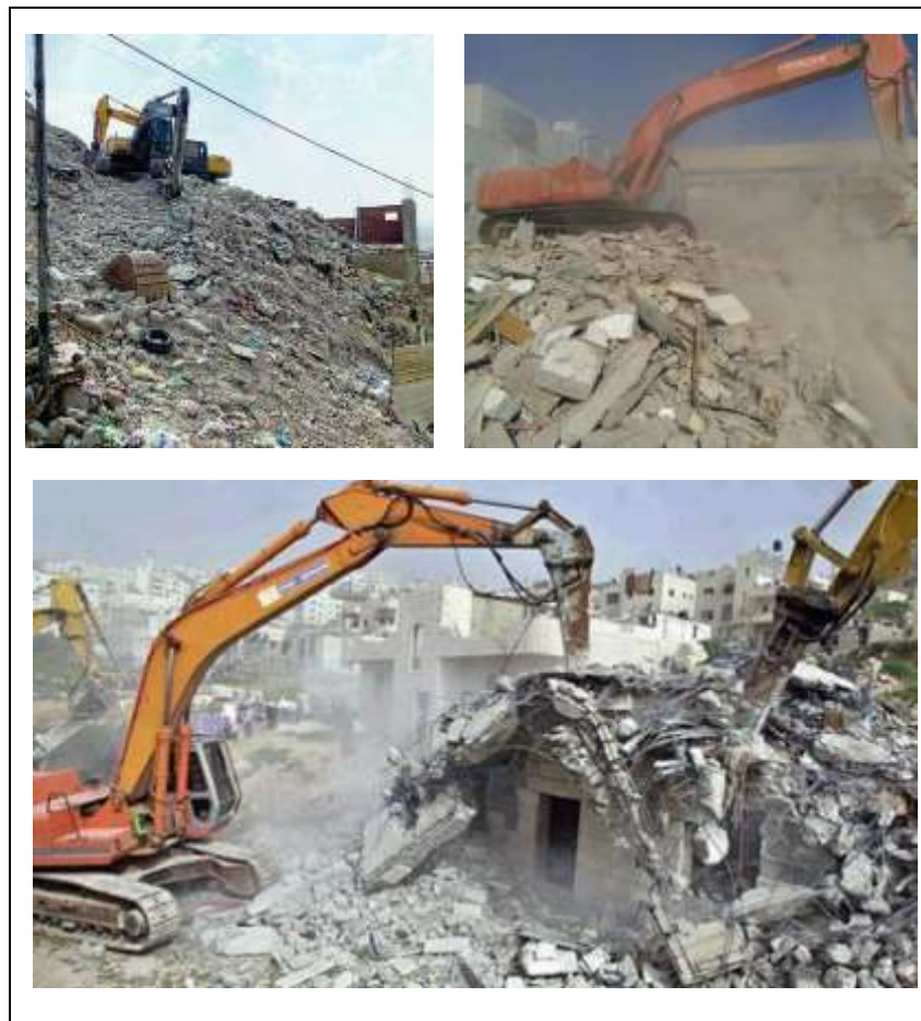
Fig. (6): Construction waste produced by demolition process in the city of Makkah – Saudi Arabia.
