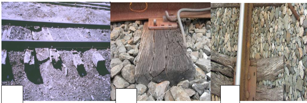
Fig.2. Types of failure modes, (a) Fungal decay [8], (b) Splitting at ends [7], (c) Spike retention[9]
