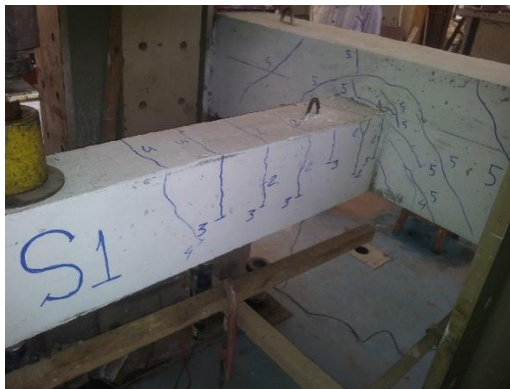
Fig. 10: Specimen-S1 crack pattern at failure
