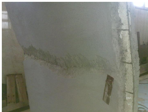
Figure 10. Failure of Wall W3
