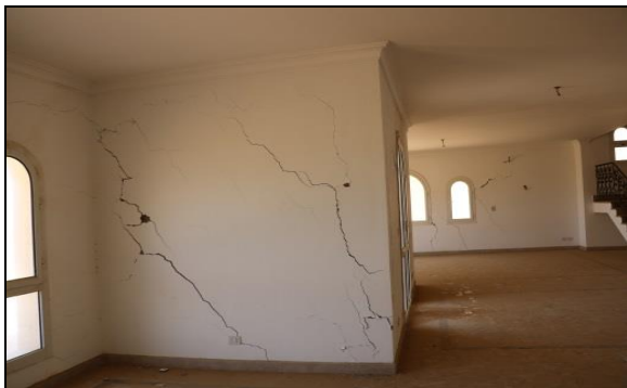
Fig. (1): Damage on a masonry wall due to soil swelling
