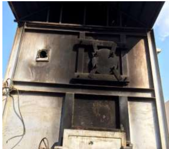
Figure 1: Incinerator frontal view
