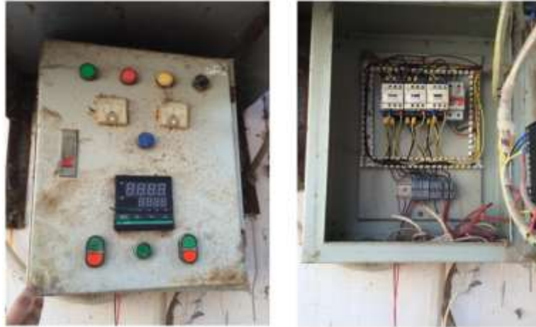
Figure 4: Outside and inside view of the control unit
