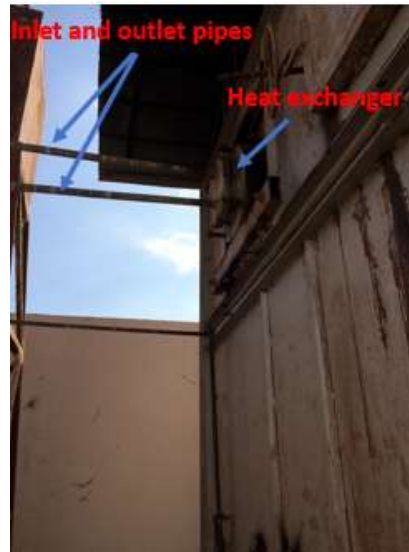
Figure 5: Incinerator with heat exchanger
