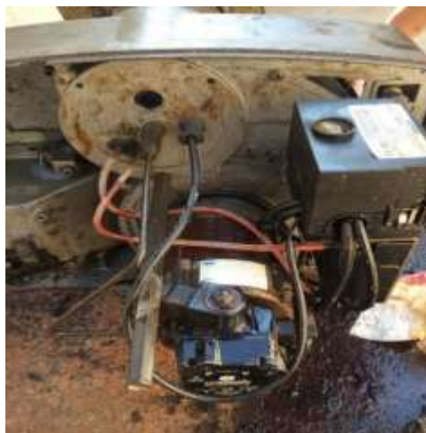
Figure 3: Internal view for the burners
