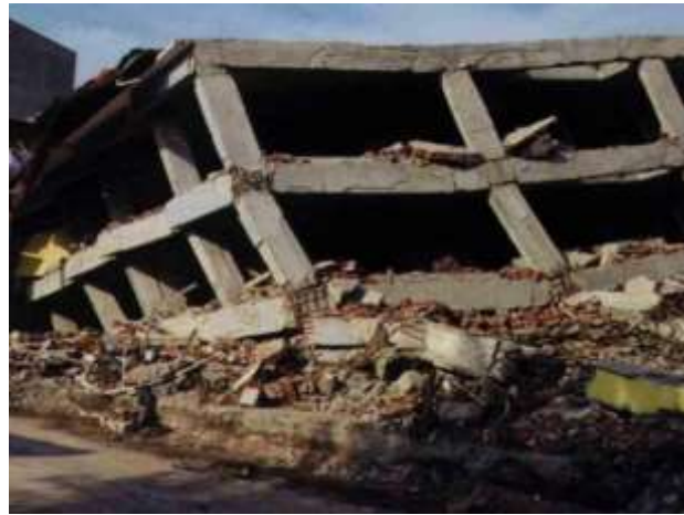
Fig. 1 Beam-column connection failure during Kocaeli earthquake, Turkey (Saatcioglu et al., 2001).
