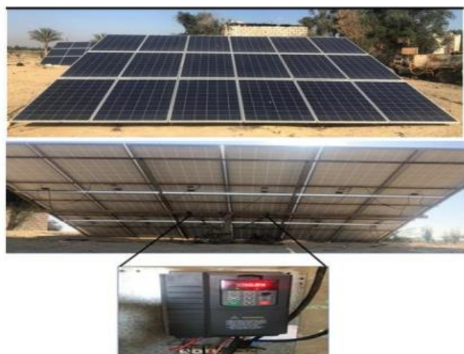
Fig. 3. Solar energy water pumping system
