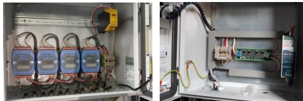
Figure 5- Voltage, current and temperature transducers
