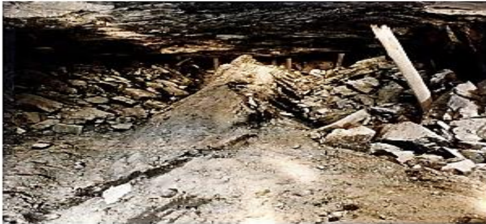
Fig. (6): Floor heave [45].
