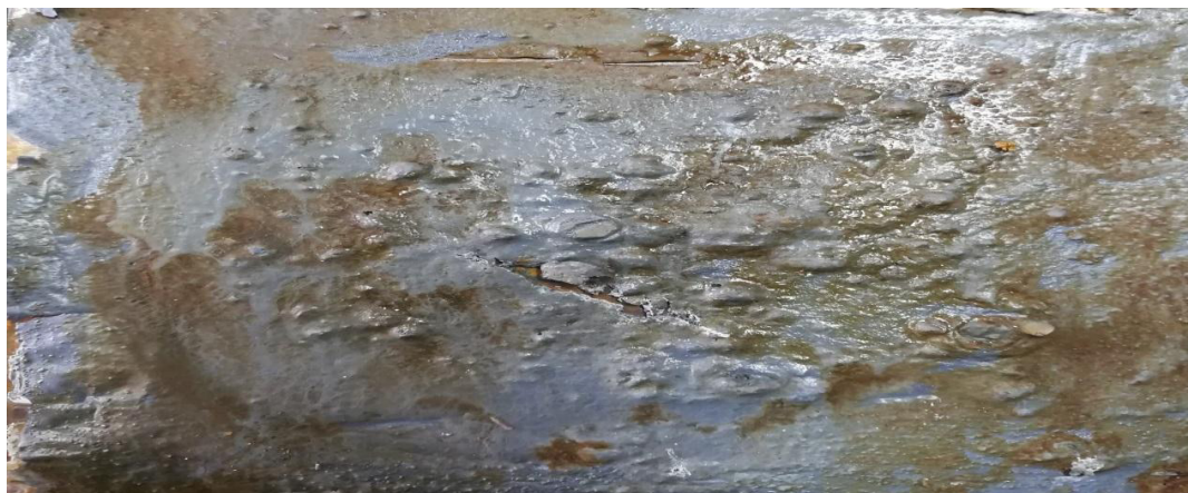
Fig. 23. Corrosion inhibitor B sample with one shell after scratching – after immersing in 10% sulfuric acid after one year.
