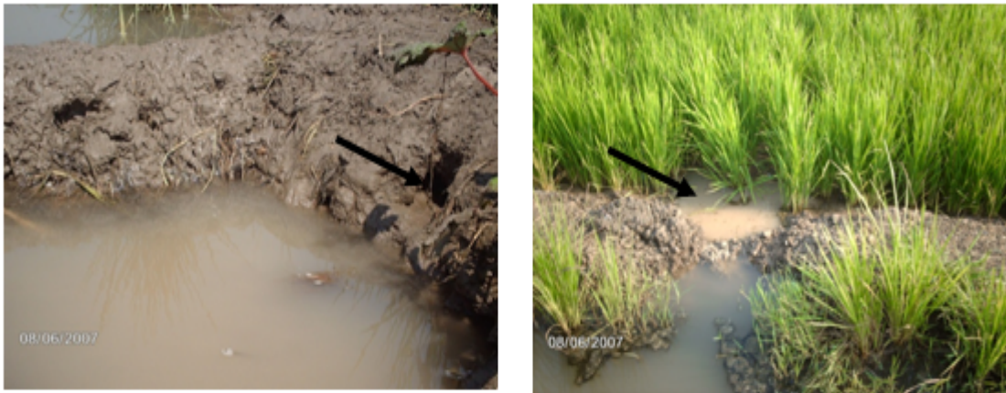
Photo 4: Damage of dykes and Rice crop in small irrigation channels at Fatmia Drain
