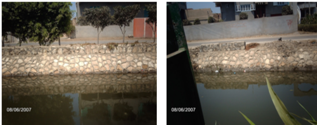
Photo 5: Pitching of damaged levees and dams of irrigation channels at Fatmia Drain
