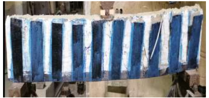
Figure 9: Tested RC beam (B3-1V-1L-15) shear failure
