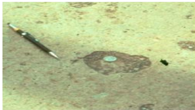
Fig.1. Scaling defect on concrete structure deck
