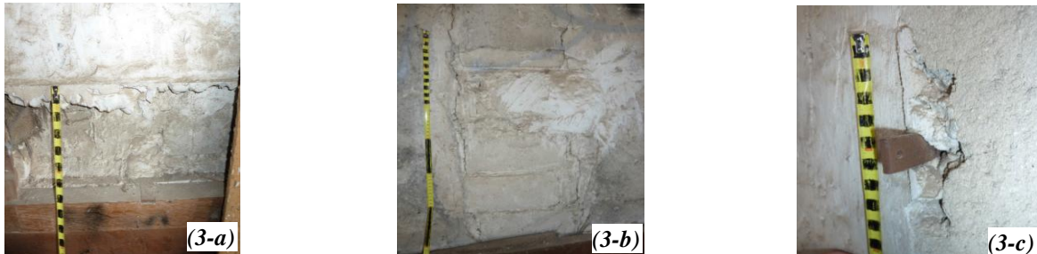
Fig. 3-a. Spalling in horizontal block. 3-b. Cracks in brick format. 3-c. Attachment wood panel and Spalling in the wall
