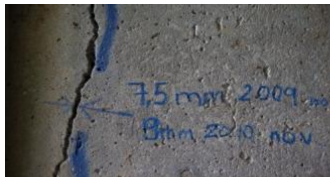
Fig.2. Crack in concrete in Turcot interchange [11].
