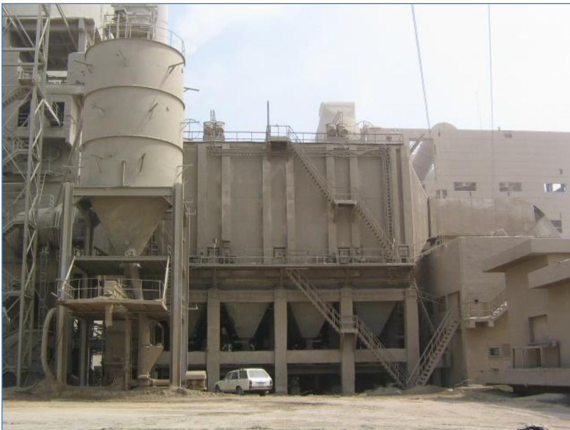
Fig. 1. The ESP in the National Cement Company.
