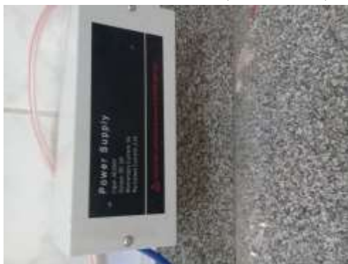
Access control power supply
