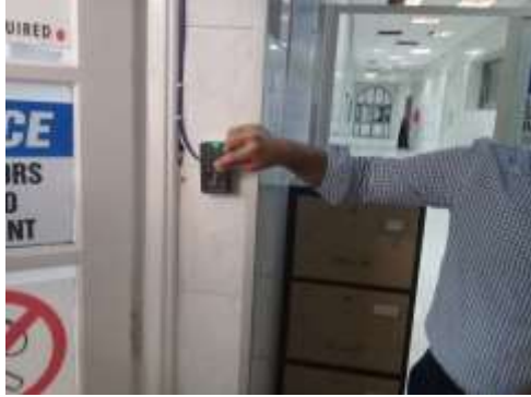
Access control (outer panel) during experimental operation of the system
