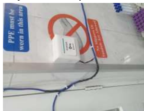
Access control push button
