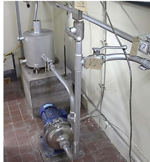
Fig. (3): Geiger-Muller and pump of purification circuit. [picture took by Beya]
