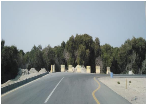
Figure 13 Construction of road networks over mangrove swamps after draining them north of Tarut Island
