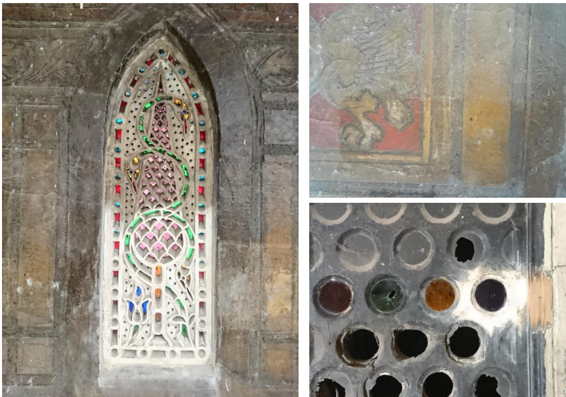
Fig 5: the lack of maintenance for the main entrance.
