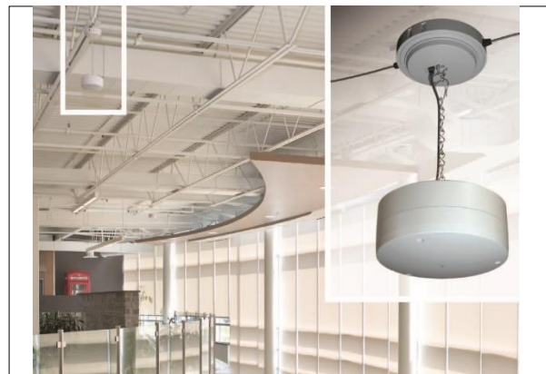
Figure 18, Sound masking system in the ceiling (Source: Niklas Moeller, 2016)
