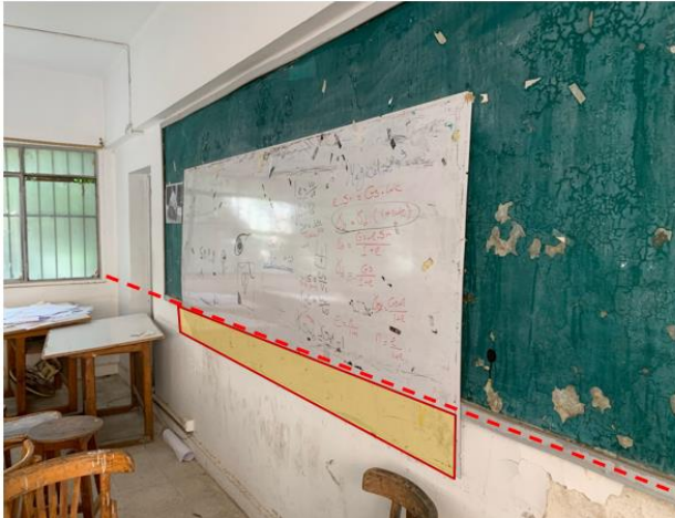
Figure 9: The chalkboard is not utilized and provided whiteboard is too small for the studio and fixed on the wrong height as from the bottom there is unused area as its on 70cm height from the floor (Source: Author)
