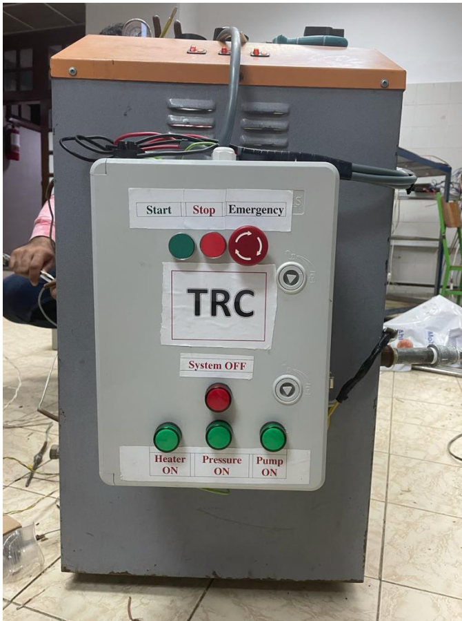
Fig. 2: The control unit
