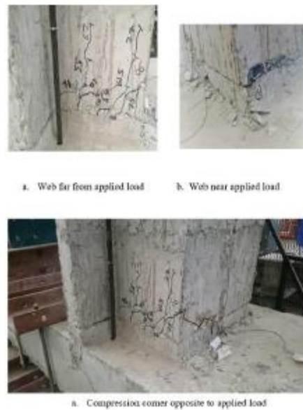
Fig. 12 Crack pattern of specimen (S2s-0.5Pys-0.2P)
