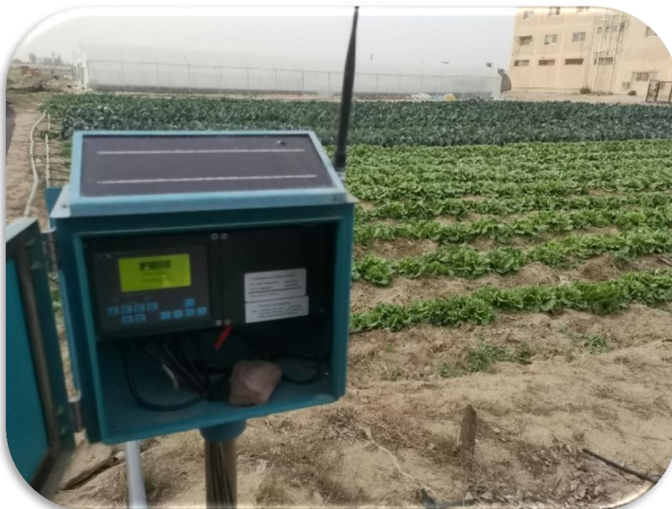
Automatic board to control of irrigation water systems
