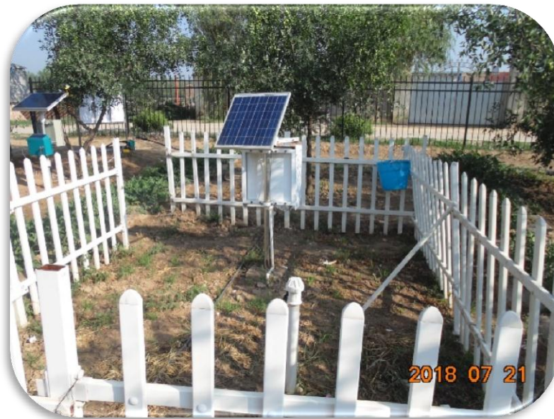
Small scale of automatic drip irrigation by solar energy
