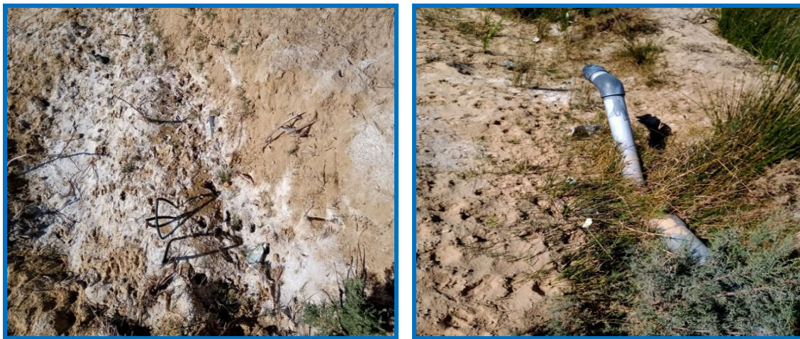
Fig. (12): Destruction of the drip irrigation network due to the desertification of the study soils
