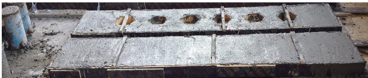
Fig.18-d. Solid and castellated beams after concrete casting. Fig. 18 Preparation and casting of solid and castellated beams.
