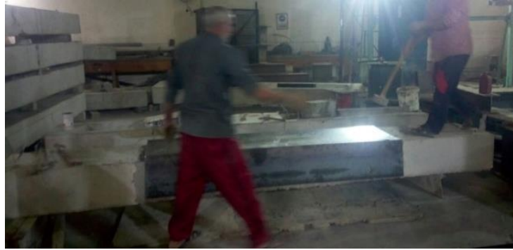
Fig. 8 Image showing the external steel plate after its application on beam B-ST.
