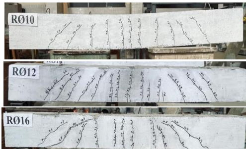
Fig. 7: Crack pattern of specimens in Group 1 at failure
