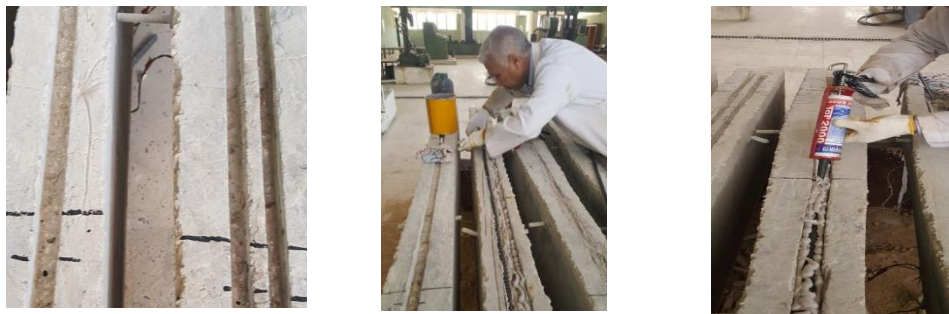
(a) After removing the wooden stick from specimens and cleaning the grooves (b) grooves filled with 2/3 epoxy adhesive and installing BFRP bars (c) filling grooves with epoxy adhesive
