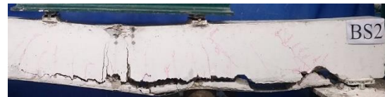
Fig. 9: failure mode of BS
