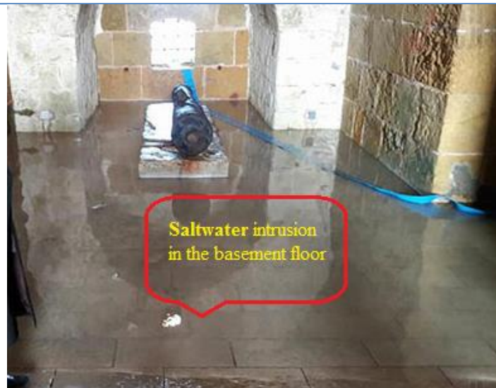
Fig (5): Saltwater intrusion inside the citadel.
