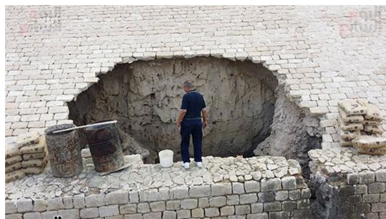
Fig (4): The hole on the northern wall of the citadel. Source: Based on photos of El-Youm El-Sabea Journal (accessed on 23, Sept 2020).
