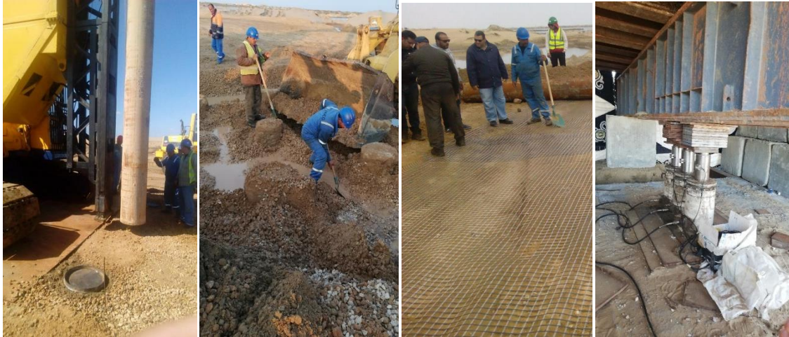
Fig. 2 Steel pipe installation, constructed RI and Geo-grid layer above the RI heads
