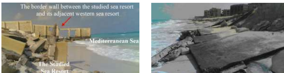
Figure 6 and Figure 7: Beach erosion of the SSR causing failure of its parallel alley and its concrete wall in 20/10/2008.
