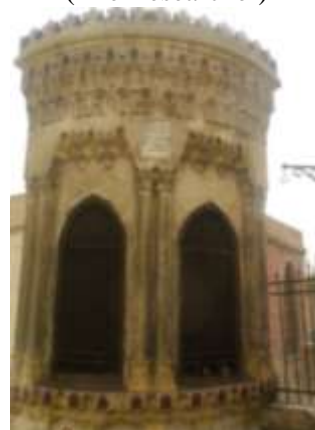
Pl. 14 The Eastern Facade of the Sabīl al-Ḥaġ Aḥmad Aḥmad al-Samāhī (The Researcher)
