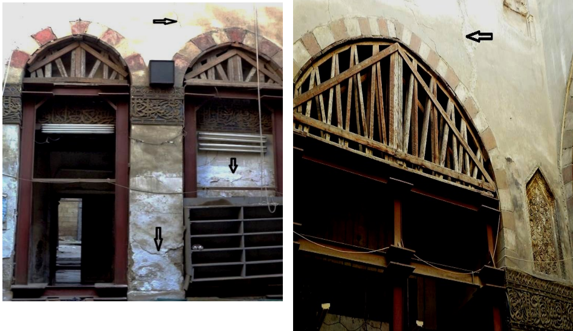
Figure 7 Tatar El Higaziya Mosque: a; The inner southern wall of the courtyard of the Mosque, b; The upper right part of the mosque's mihrab wall, showing High humidity in the inner walls of the mosque and the deep cracks salt efflorescence and wrong restoration by native people (arrows).
