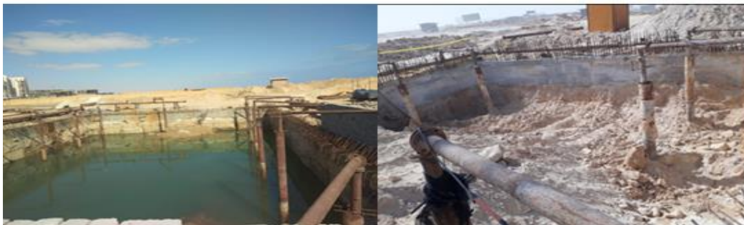
Fig 11: Leakage from weak points in diaphragm walls during excavation
