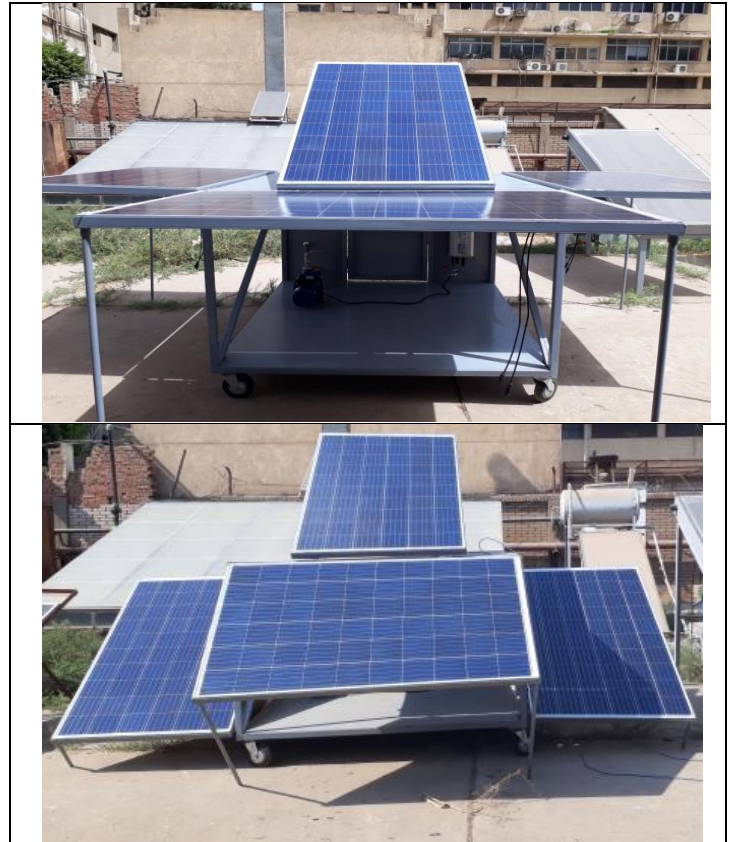
Fig. 3: Photographic view of the studied PV system
