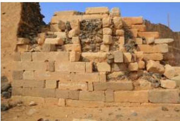
Fig:15 Coherence of architecture at the confluence of the two walls (A) and (B).
