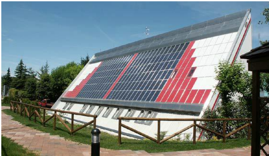
FIG 8: PV combined with a thermal system (PVT) façade of Fiat Research Center
