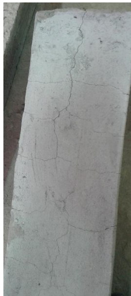
Cracks Appeared in post-heated column C2
