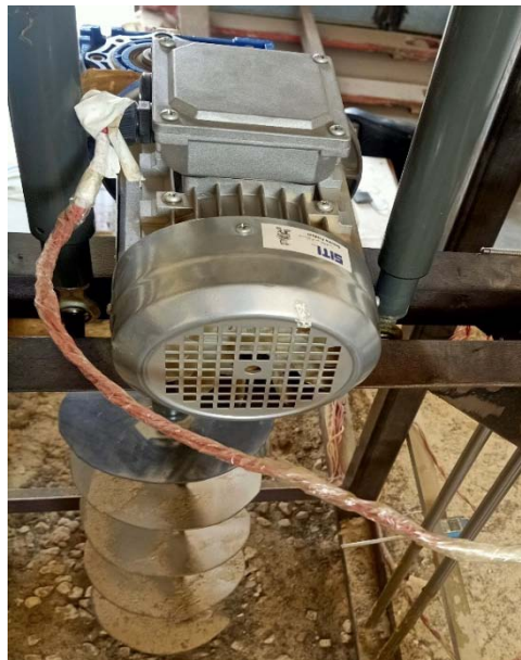
Figure 11. A three phase AC motor.
