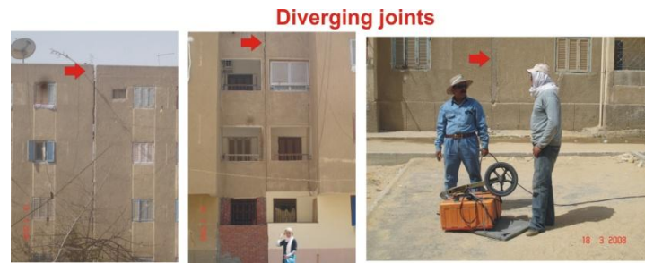
Fig. 2: Photograph for some deformation appearances as a result of foundation instability.
