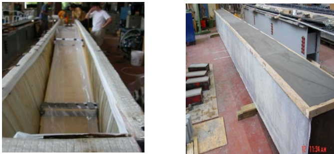
Fig. (3): Detail of interior and exterior engineering design of HCB composite structure.
