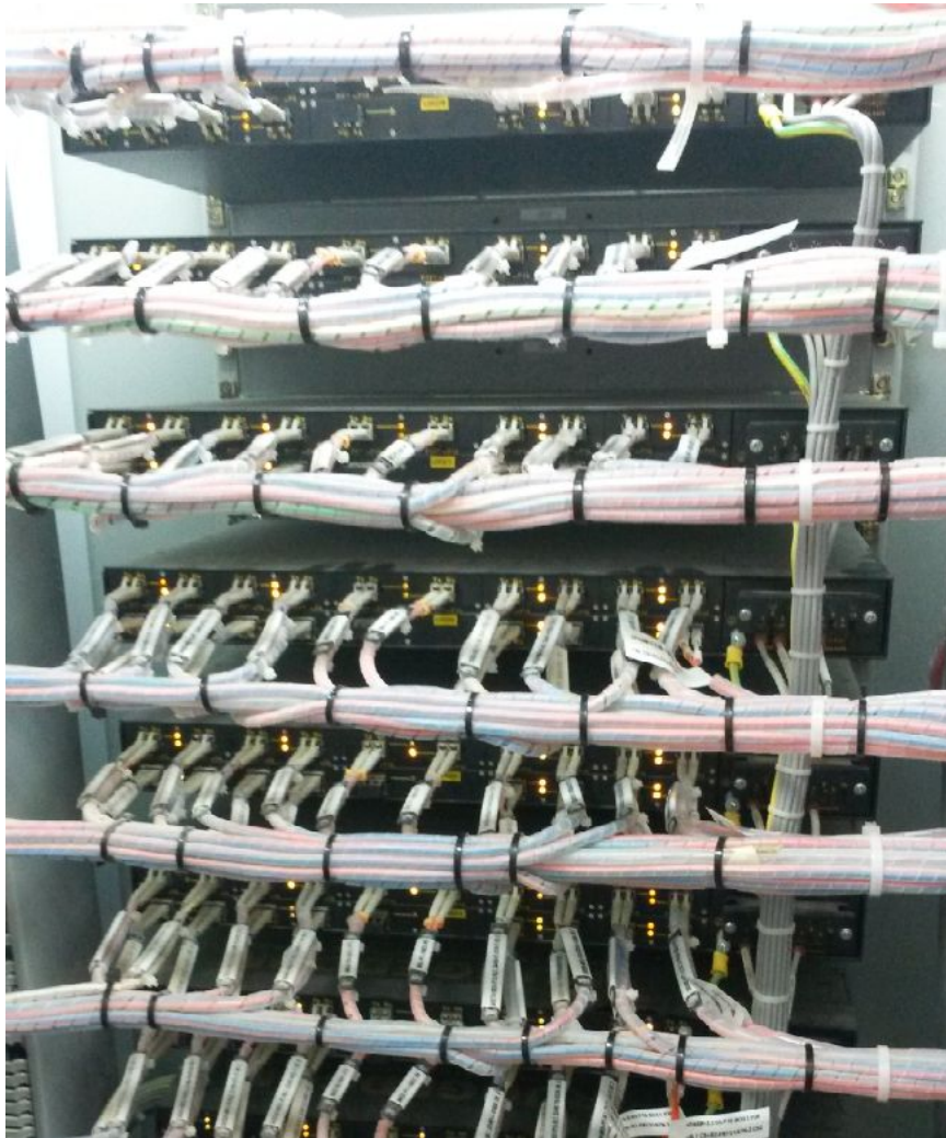
Figure (4): Communication units with protection relay
