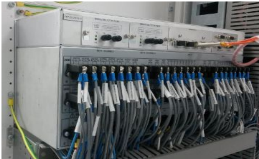
Figure (3): Protection relay connected by fiber with the communication unit
