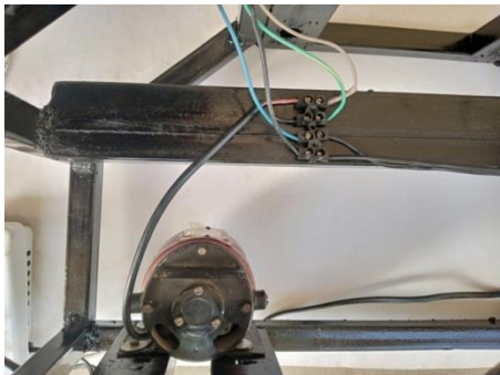
Plate 7: Inserting a Connector as the central point of all connections to avoid electricity shock during operation
