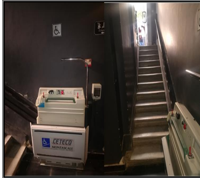
Fig.75. Device as access ramp for Physical Impaired facilities, (researcher picture)
