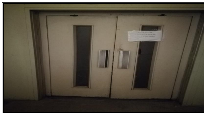
Fig.87. Elevator for Physical Impaired facilities, (researcher picture)
