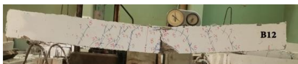
Fig. 11 Pattern of cracks of beam (W2).
