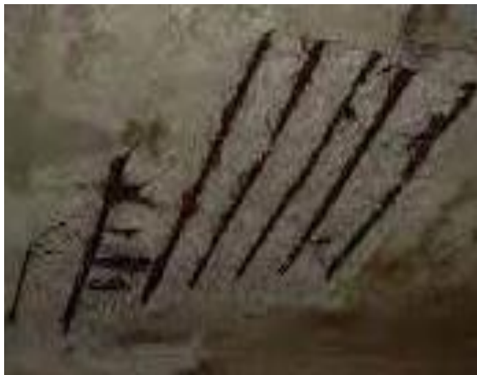
Fig. 1 Corrosion of steel bars.
