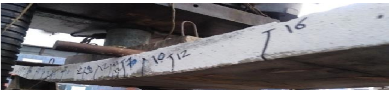
Fig. 12: Crack pattern for RC slab, S-St-BF-zero%-Ext.
