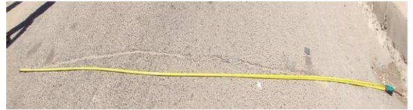
Fig. 5. Transverse crack No.4.
