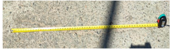
Fig. 4. Longitudinal crack No.3.
