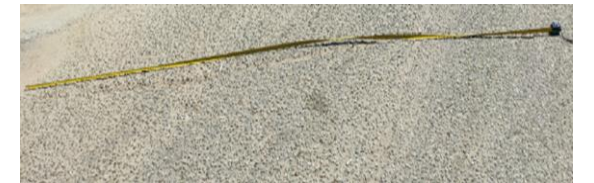
Fig. 7. Transverse crack No.6.
