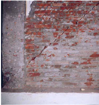
Figure 1 Failed in filled frame with a prominent diagonal crack [8].
